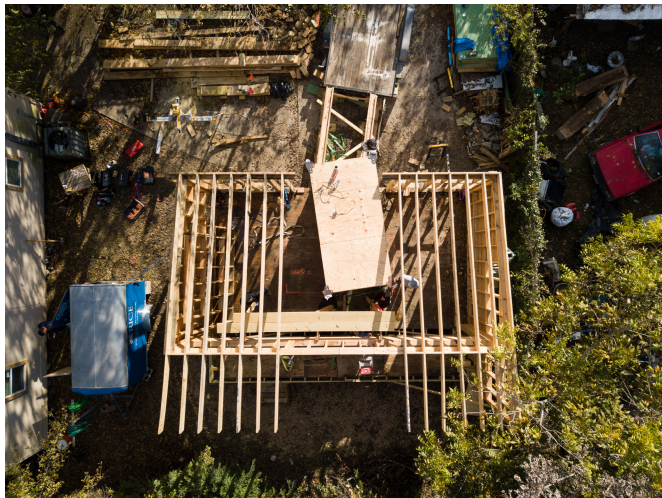
Figure 1. Introduction of the prefabricated core during construction of +House. The project was developed as Rice Building Workshop transitioned to become Rice Architecture Construct and is the program's first completed Accessory Dwelling Unit.
