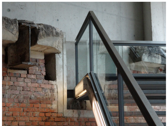
Figure 4: The corner of the stairs cutting into the existing brick wall. Photo by Author.
